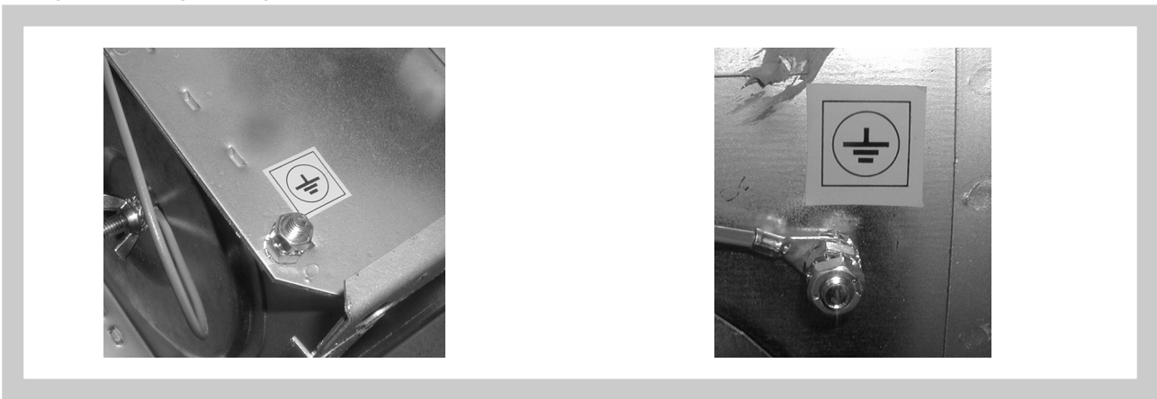
Fig. 4 The grounding screw on the fire damper
